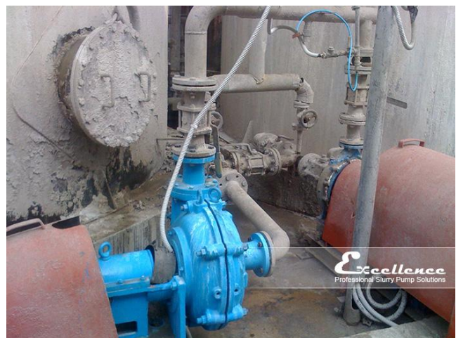
50EZ-A50 in Mid-East Sodium Silicate Plant
