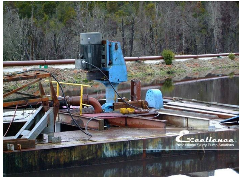
EVHM-6SV in Coal Washery in Australia
